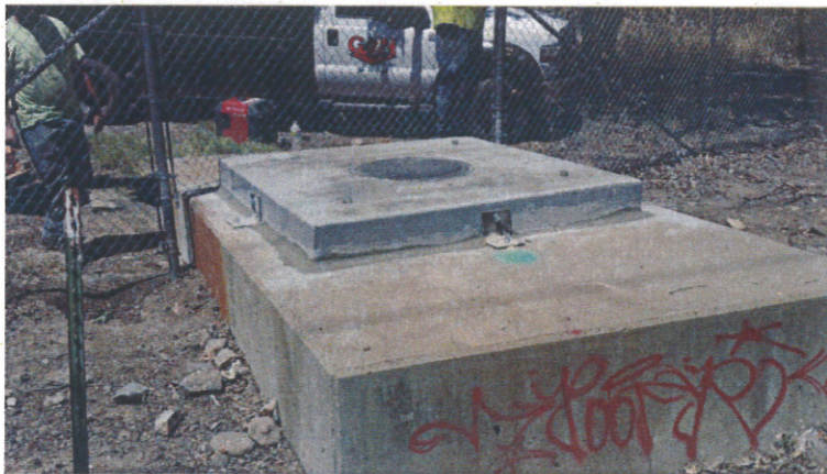
Van Buskirk Inlet Vault- Air Tight Cover
