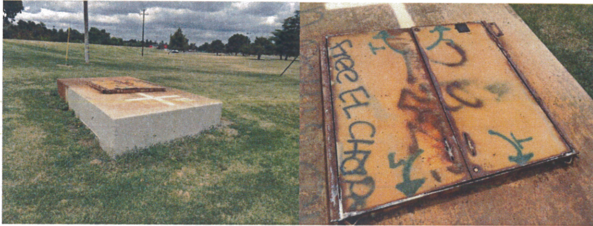
Van Buskirk Outlet Vault-Corroded Cover
