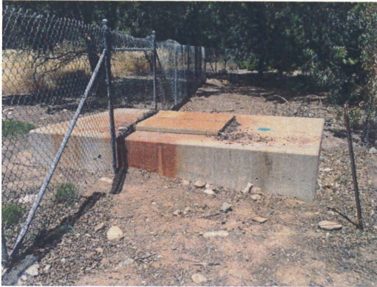
Van Buskirk Inlet Vault- Corroded Cover
