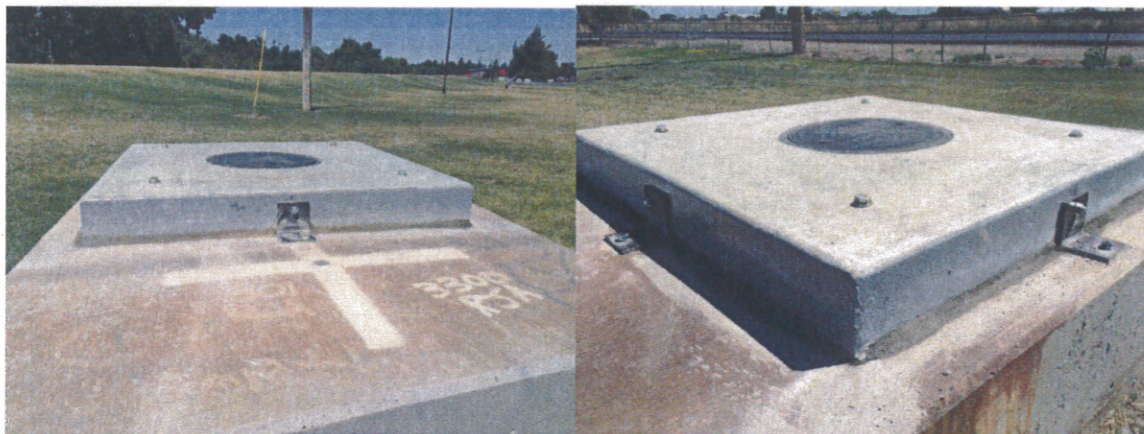
Van Buskirk Outlet Vault- Air Tight Cover
