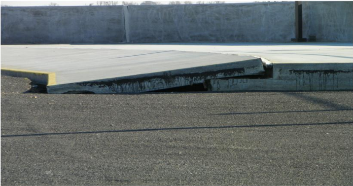
A concrete slab has shifted due to soil settling at the IPS.
