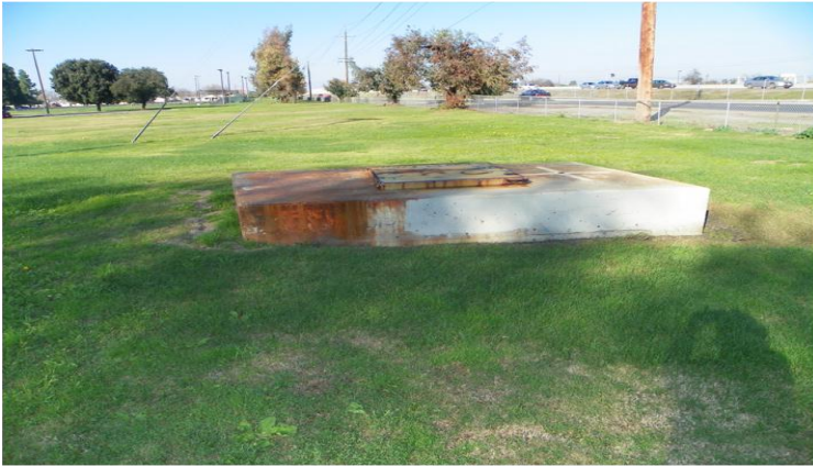
A utility vault at Van Buskirk Park with a cyclone fence in the background. Both show signs of corrosion.
