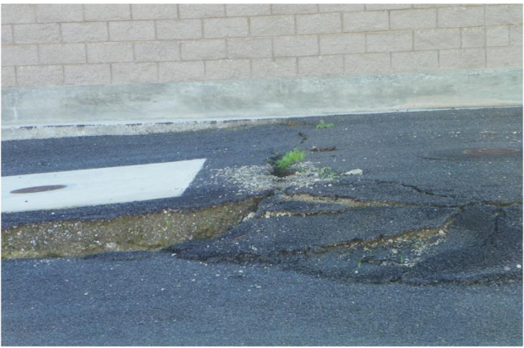
Buckled asphalt at the IPS because of soil settling.
