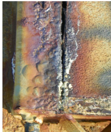
Photos above and at the right are close-ups of corrosion on the two-year-old utility vault doors in Van Buskirk Park.
